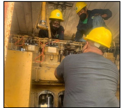
Work in progress to resolve faulty generation unit supplying power to Caye Caulker.
